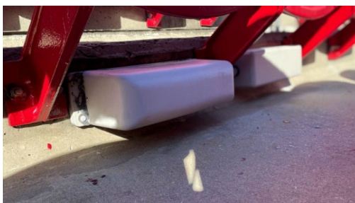
Fig 8-1 5G millimeter wave small cell installed under the seat of the stadium
