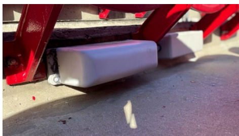
Fig 8-1 5G millimeter wave small cell installed under the seat of the stadium
